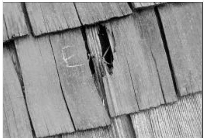
Figure 8. Eroded opening in a cedar shake.
