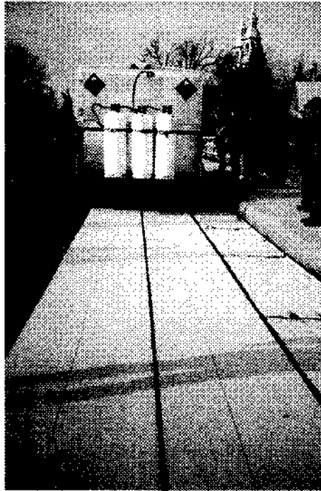
Photo 6: The machine unrolls, welds and presses down on the membrane in a single pass
