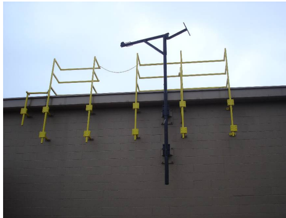
Integrated guardrails for permanent equipment hoist
