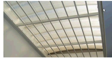
Exterior and interior skylight fall protection
