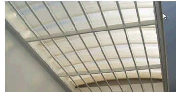
Exterior and interior skylight fall protection
