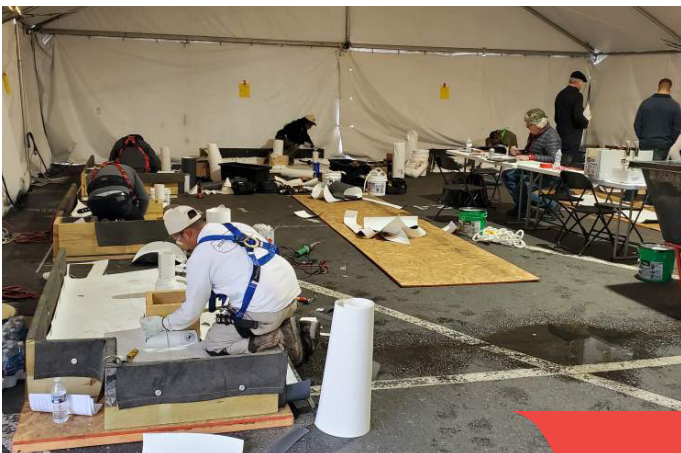
NRCA ProCertification® on-site testing at NRCA's 133rd Annual Convention and the 2020 International Roofing Expo®
