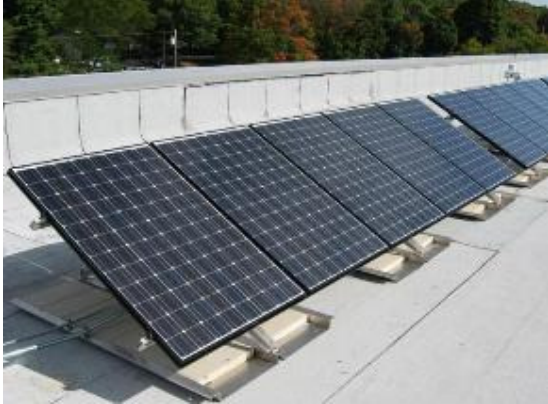
Figure 6: Representative ballasted low-slope roof system installation (picture taken from ( http://www.altpowerinternational.com/solar-pv/installations.php ))
