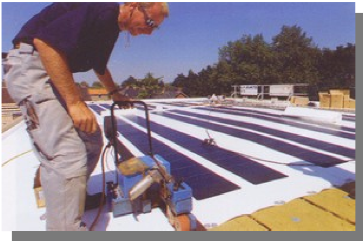
Figure 7: Application of a low-slope roof membrane which incorporates pre-laminated flexible PV modules
